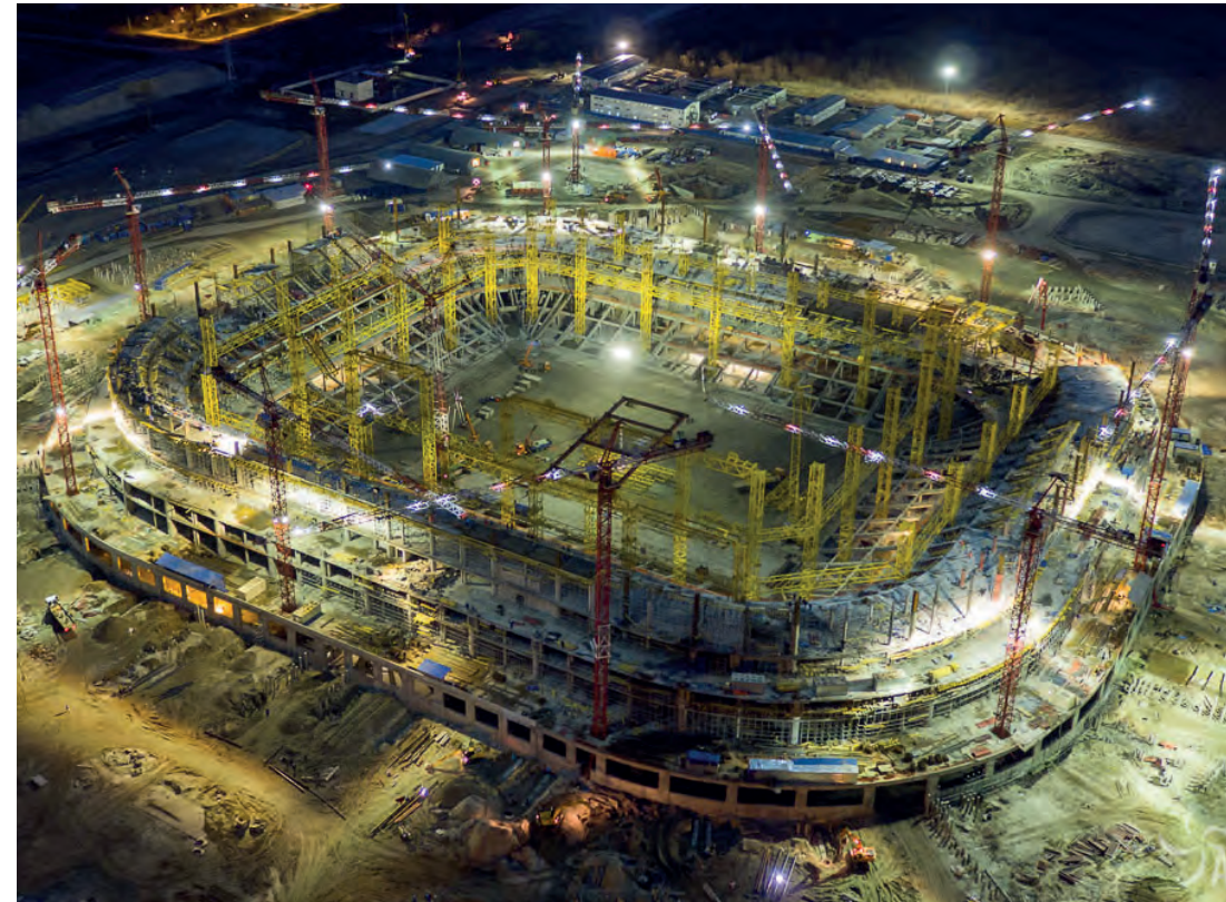
Rostov Arena in Russia; photo at night of the Football Stadium under construction. This is one of the venues for the 2018 FIFA World Cup.
