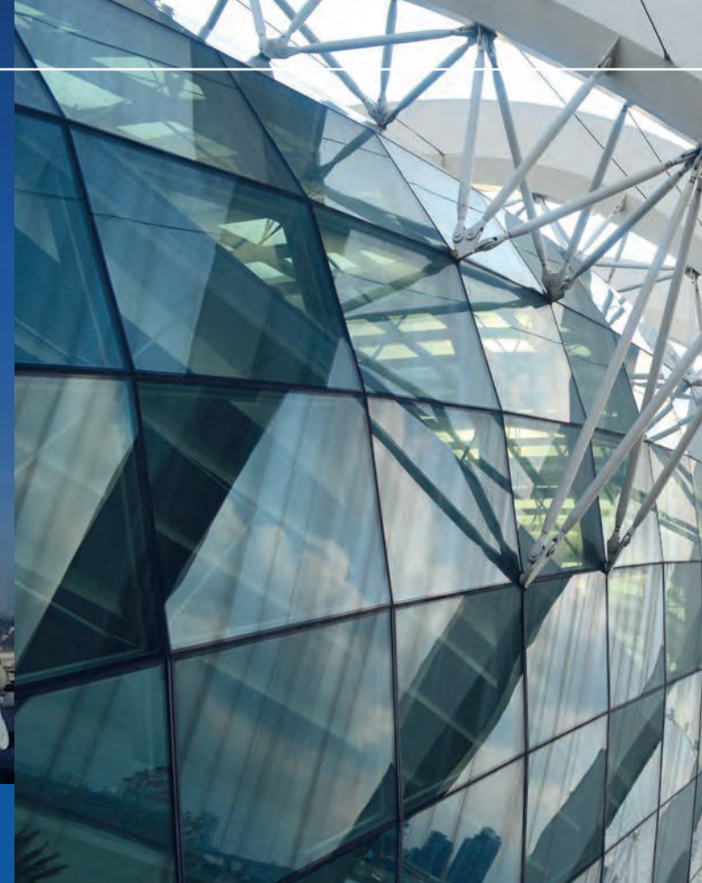
City Deco Prague utilising Macalloy Tension Bars to assist in supporting the office building structure
